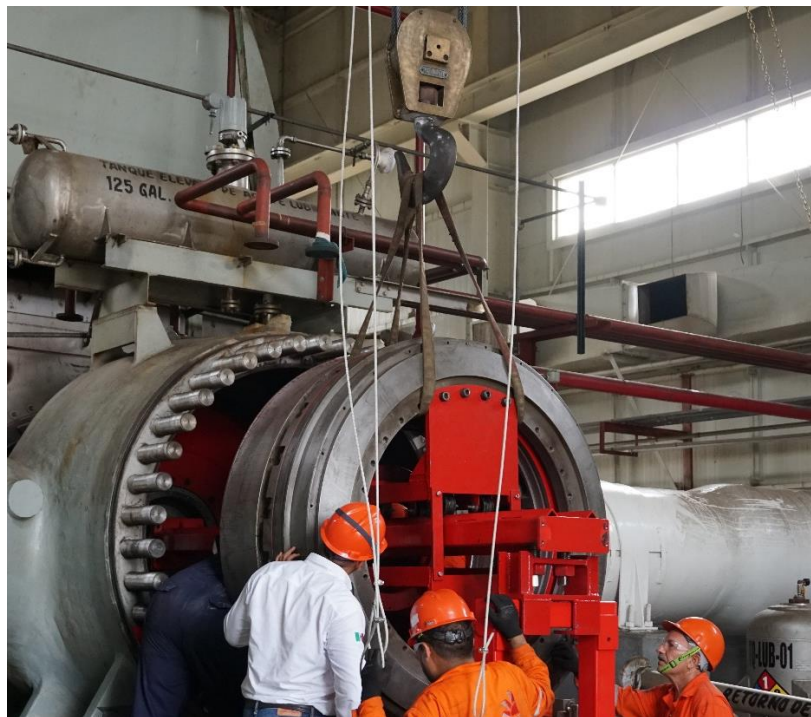
Rolls Royce – Cooper RF2BB-36 Compressor Installation
